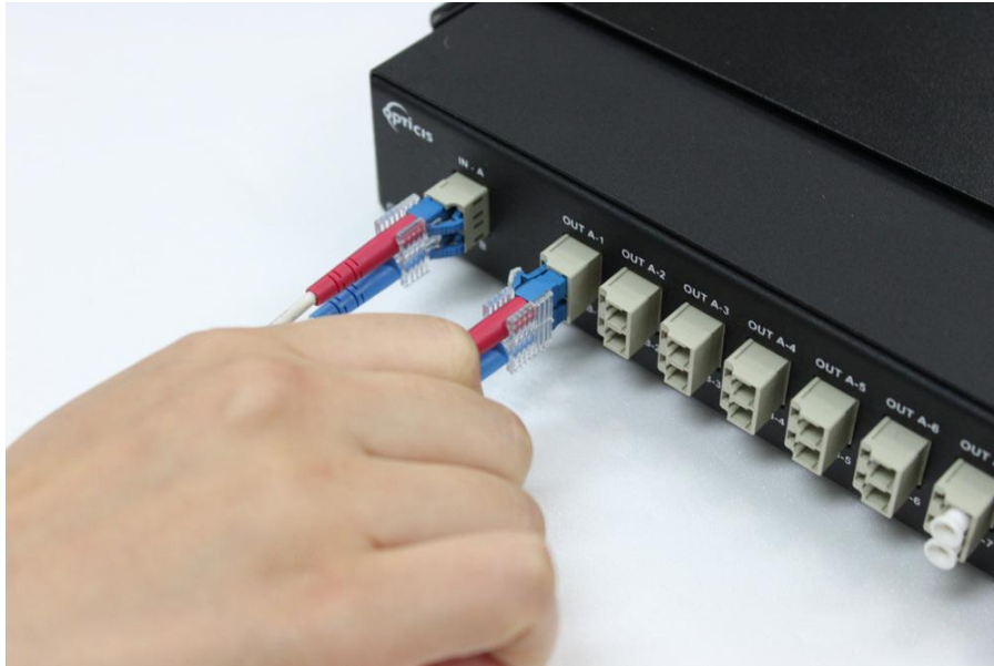
Fig. 8: LC patch cord into output receptacle
